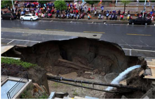
(a) Road collapse in Jiangsu
