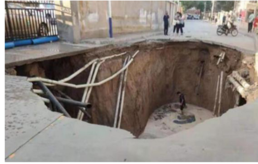
(b) Road collapse in Lanzhou
